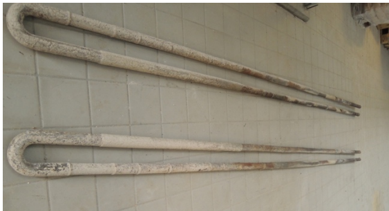
Figure 9. Photo showing of two of the three Steamboost tubes removed from the boiler
