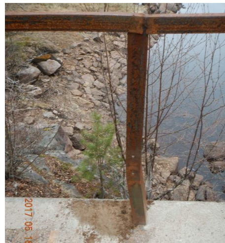
Räcke – deformation, korrosion
