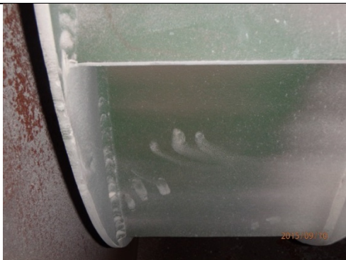
Figure 58. The flue gas fan at inspection 2015
