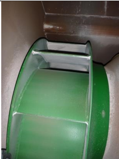
Figure 57. The flue gas fan at inspection 2014
