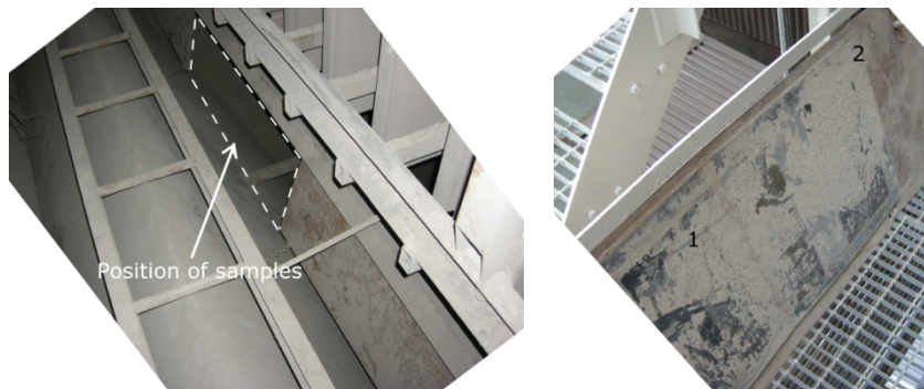
Figure 46. Photographs showing the position of the samples in the electrostatic filter (arrowed, left) and the two sample panels removed from their position (right). While the panel marked "1" was brushed slightly after removal, the deposits of the samples are clearly observed in the panel marked "2".
