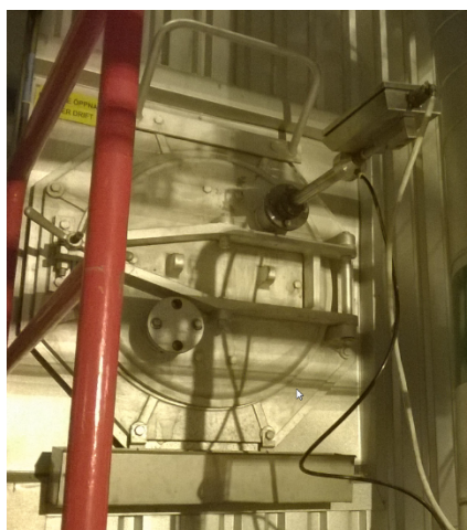
Figure 115. Online corrosion probe installed in Händelö P15 boiler empty pass during the campaign 3.
