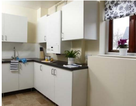
Combined Heat & Power (CHP)
