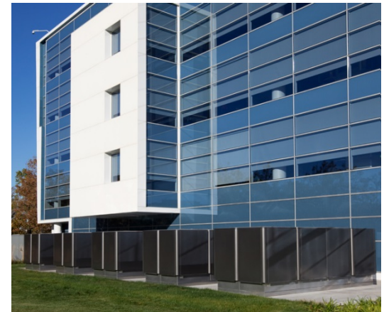
Off-grid power generation
