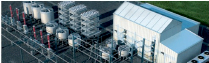
STATIC SYNCHRONOUS COMPENSATOR (STATCOM)
