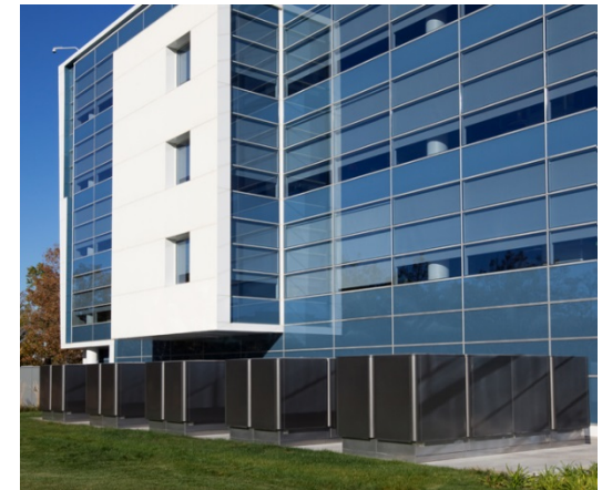
Off-grid power generation
