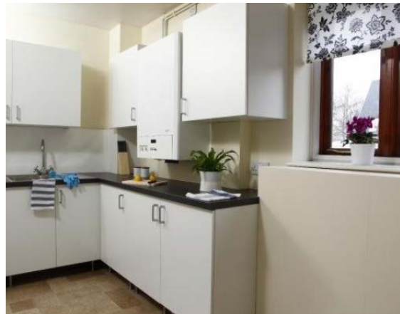
Combined Heat & Power (CHP)
