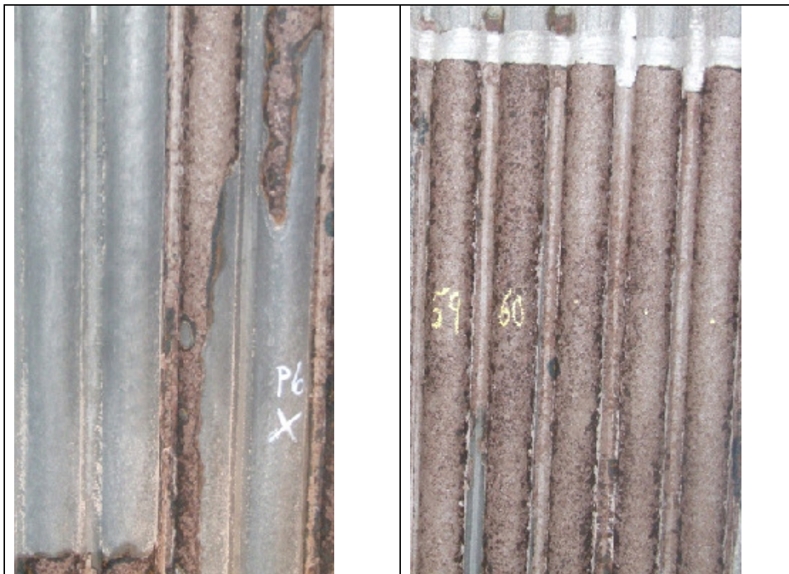
Figure 10 Sample P6: TP316 stainless steel coating plasma-sprayed in workshop by MH Engineering and installed in the boiler in summer 2011. Large areas had delaminated and were missing, but the remaining area was in good condition. The coating was applied on tubes 59, 60, 62 and 63. The sample was taken from tube number 60.
