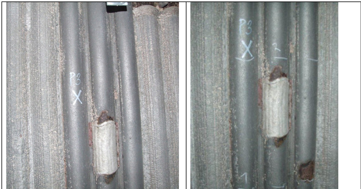
Figure 7 Sample P3: Alloy C-276 Flame Spray. The coating was applied in summer 2008 on tubes 52-54. The sample was taken from tube number 52.
