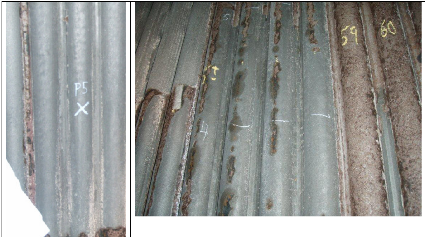
Figure 9 Sample P5: HS4 coating plasma sprayed in workshop by Häuser and installed in the boiler in 2011. The coating was severely damaged in some areas. The sample was taken from tube number 56. The coating was applied on tubes 55-58.
