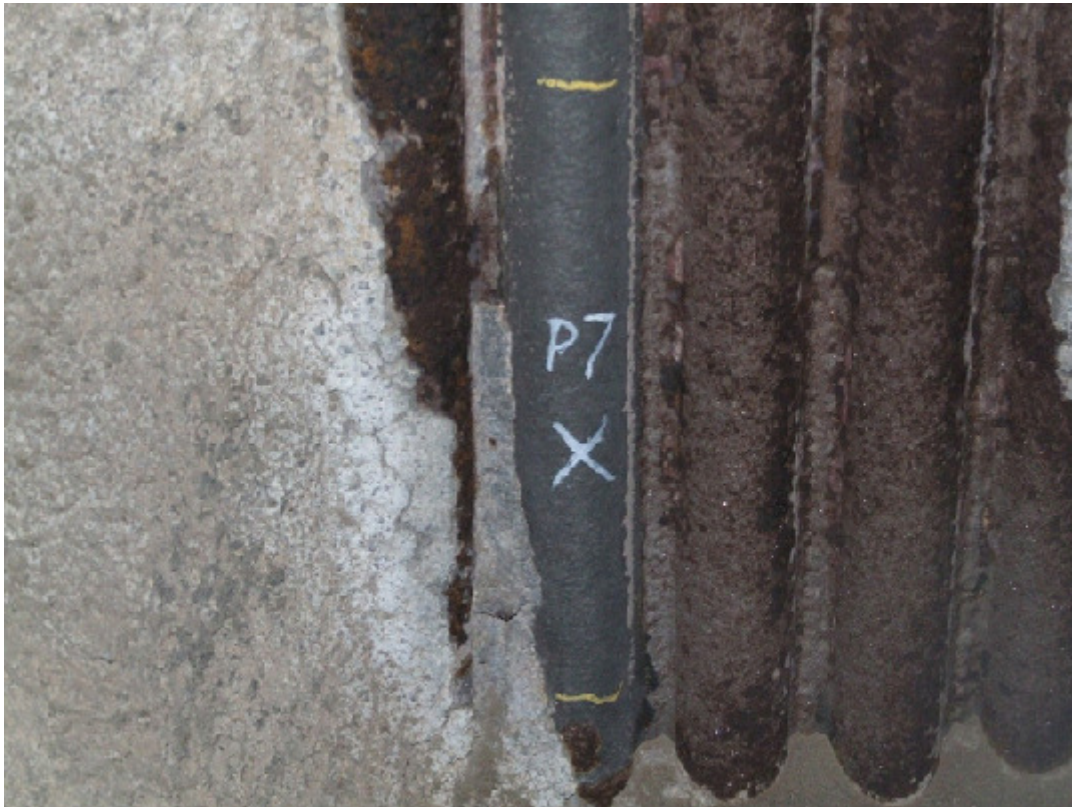
Figure 11 Sample P7: CorrEr The coating (only one tube) was applied during summer 2011 by MH engineering on site. The coating had delaminated at the top. The sample was taken from tube number 65.
