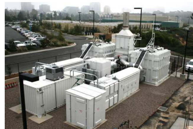
STATIONARY (2015-2016) 0,5kW – 3 MW
