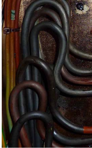
Excessive bending stresses on cable installation
