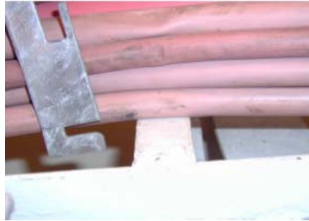
Poor clamp design producing excessive compressive forces on cables
