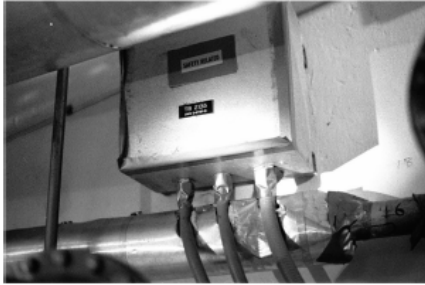
Displaced thermal insulation on valve operator
