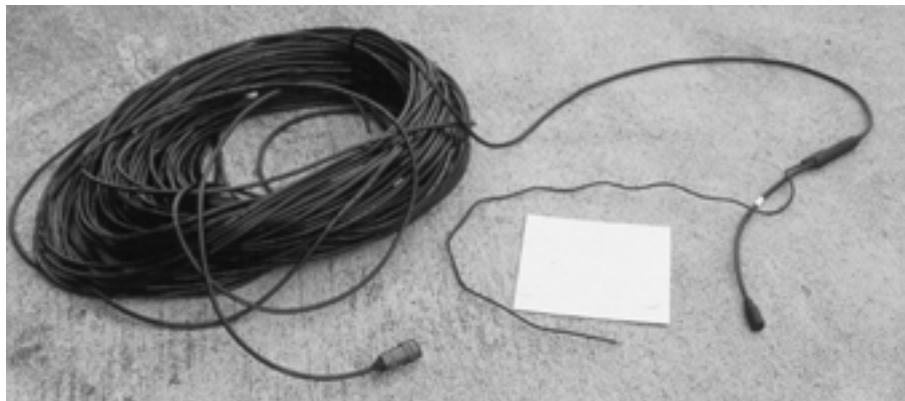
Figure 2-3: Electrode and multi-core cable used on the dam crest and the downstream toe.
