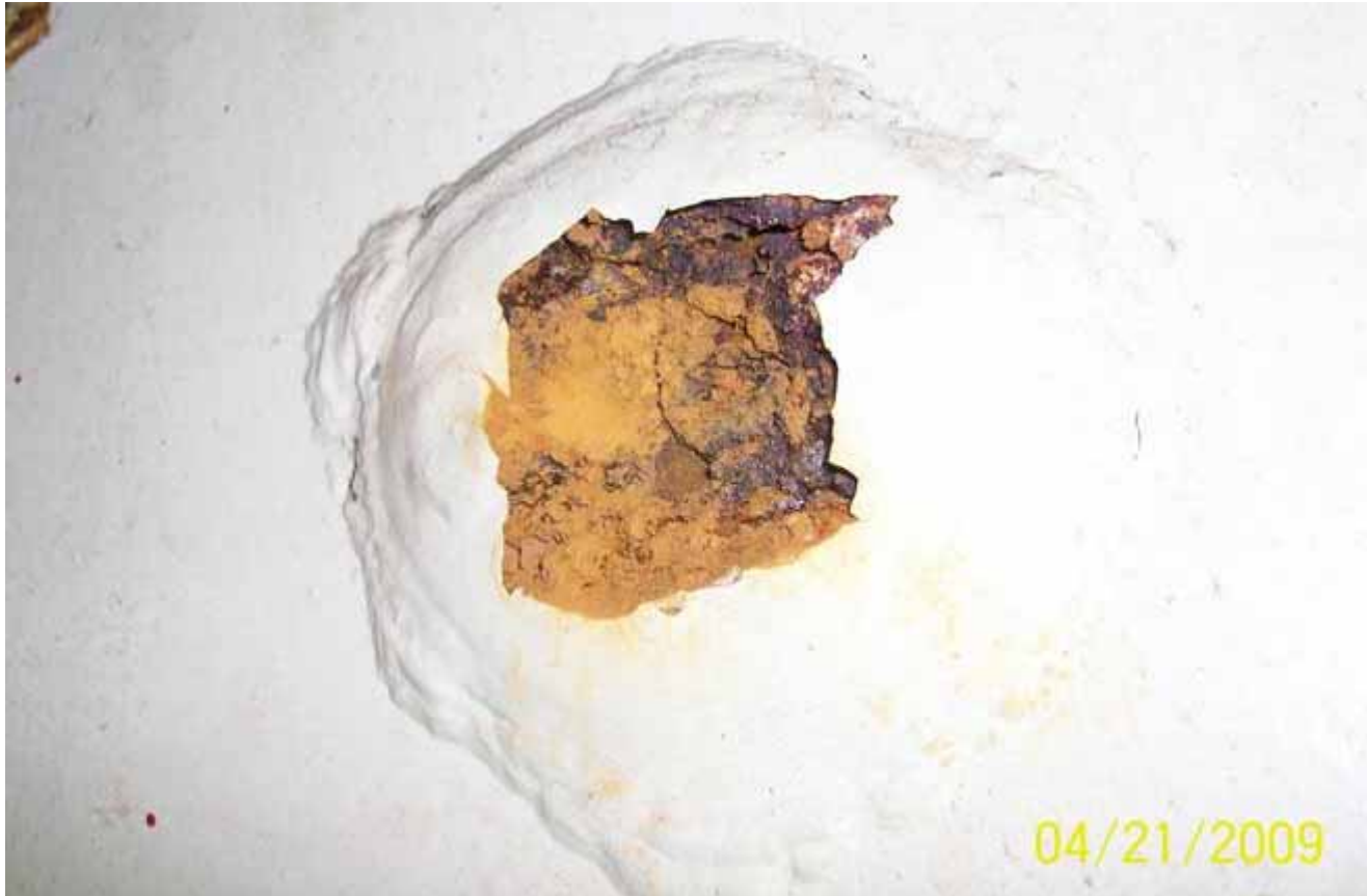
Paint Blister with Corrosion Products Identified at Beaver Valley Unit 1 in 2009 (FirstEnergy, 2009).
