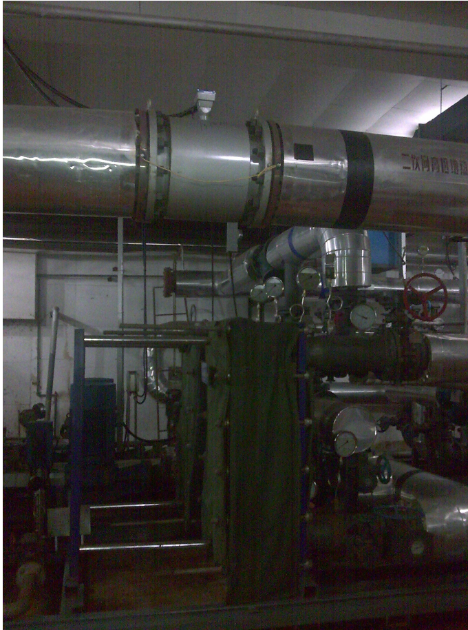
Picture 12. Substation view with heat exchangers for one residential area and the flow meter installed in the pipe above.
