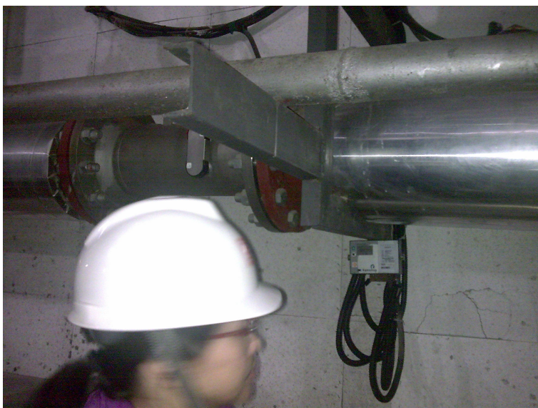
Picture 11. Mei Gong checking the installed heat and flow meters in the substation.
