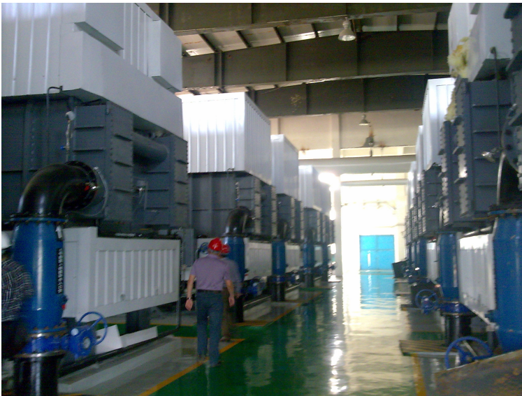
Picture 14. Interior picture from the heat pump station containing six large absorption heat pumps with a total capacity of 225 MW.
