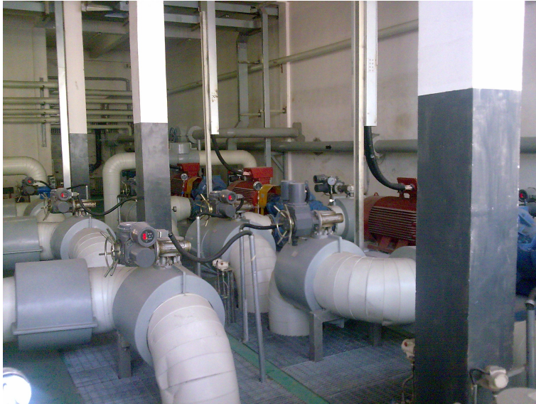
Picture 10. Pumps and valves installed in the pumping station.
